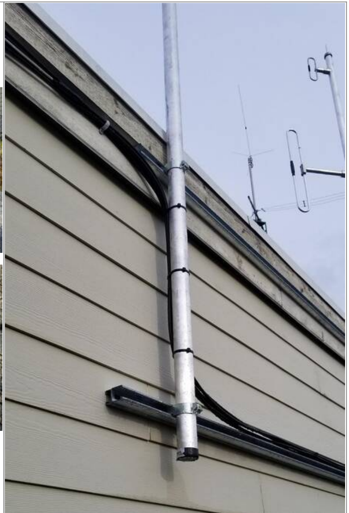
Wall mounted using Unistrut channel.
